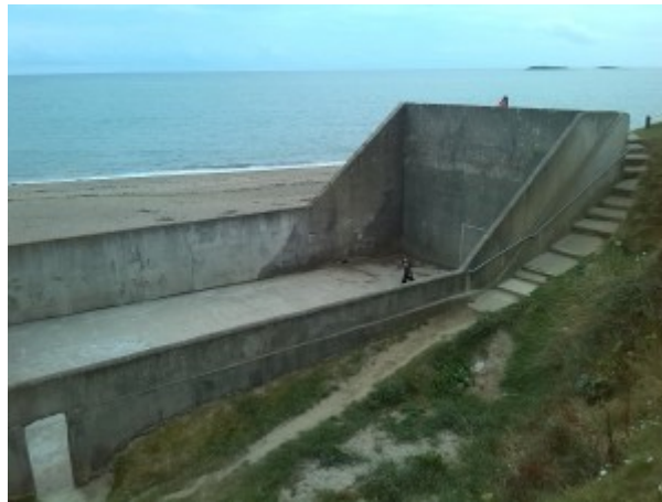
A side view of the court showing the famed steps going up to the top of the front wall
